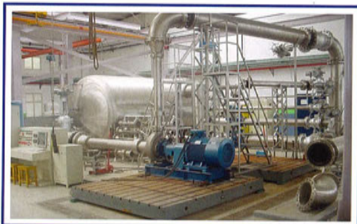
Test bay at the factory
